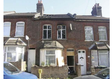
Lot 59 – Fire Damaged House
